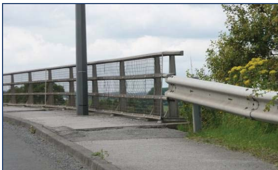
② Evidence of footway subsidence on embankment
